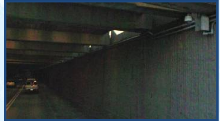
Dome Camera in Dorval Tunnel
