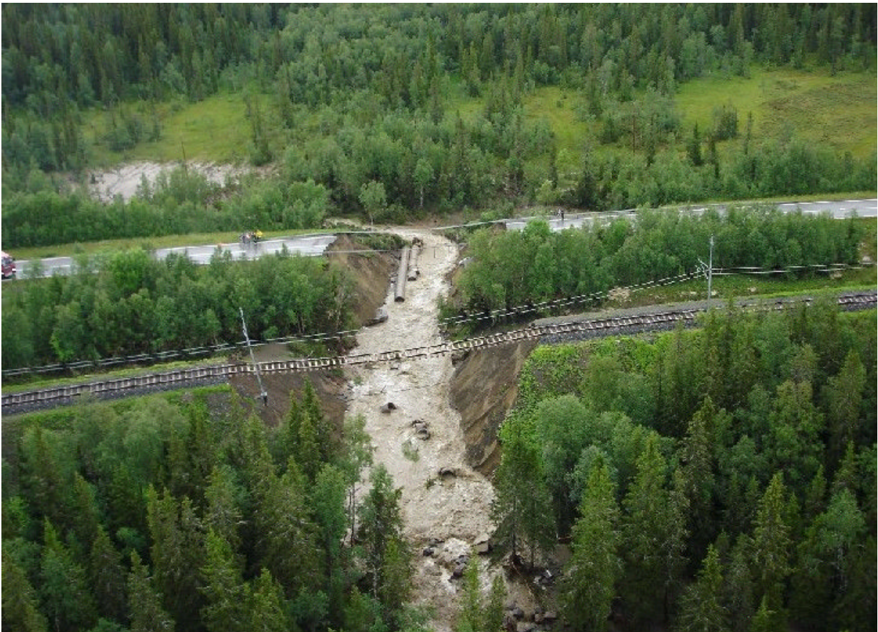
Landslide at Enafors, Jämtland, 2006
