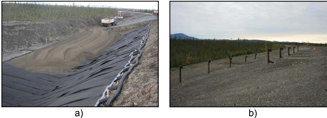
Figure 4 – a) Backfilling over geocomposite on slope heat drain section. b) View of finished heat drains with insulation section.
