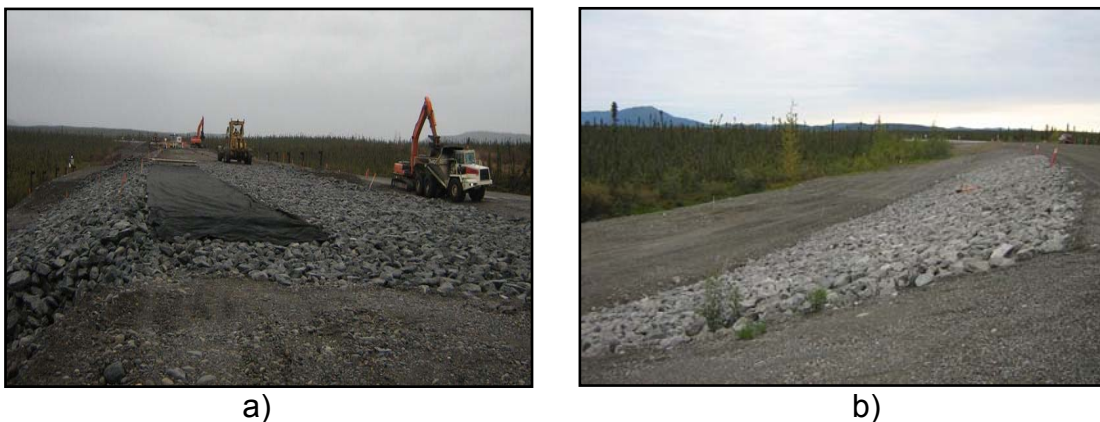
Figure 3 – a) Full ACE embankment built; placing geotextile prior to base course. b) Finished uncovered ACE slopes section.
