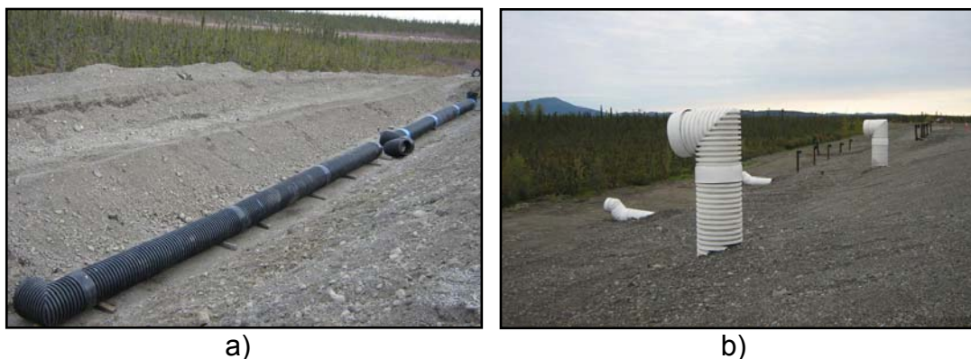
Figure 5 – a) Longitudinal culverts placed in trench with some heat shrinking complete (blue joints) and prior to heat shrinking and backfill. b) Finished longitudinal culverts showing inlets (horizontal pipes) and outlets (upright pipes).
