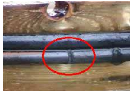
Fig.8-Failure test on cabling
