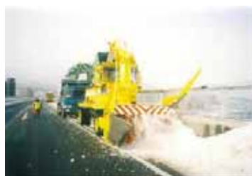
c. Snow hauling operations on the elevated section Photo 3-Scenes of snow piled on the shoulder and snow being hauled away
