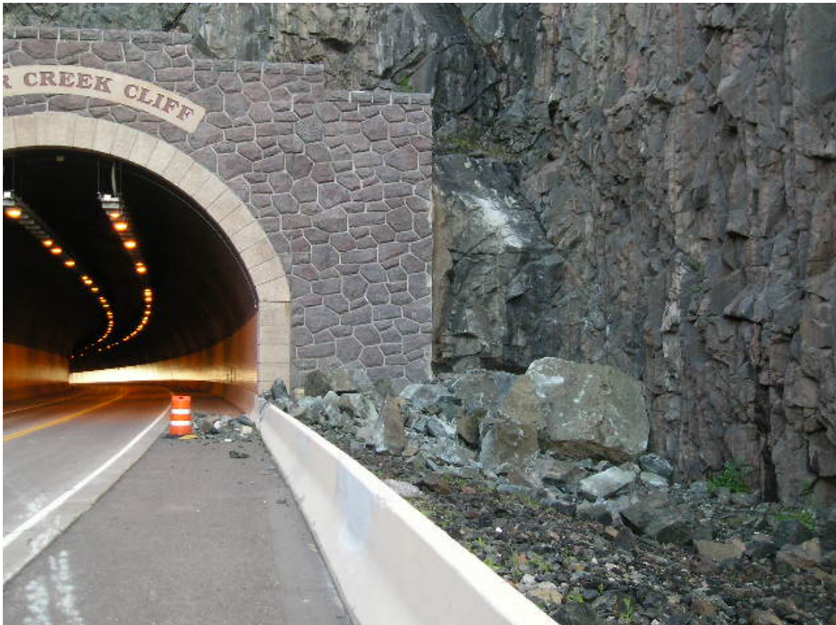
Figure 2. Rock Fall debris at Silver Creek Cliff Tunnel on Minnesota Trunk Highway
