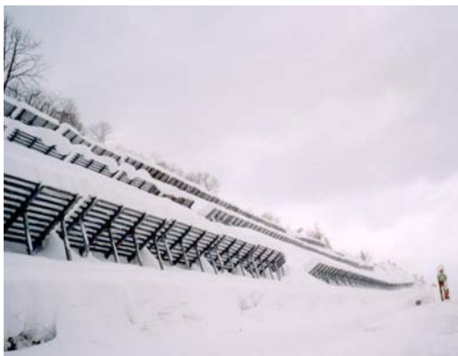
Snowslide protection fence
